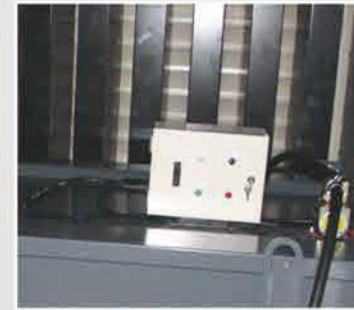
Automatic fueling device
