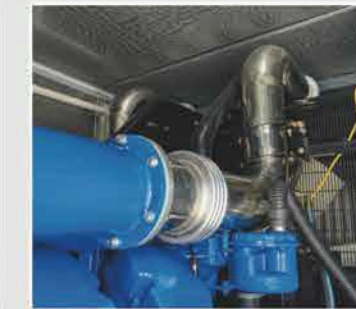
Interior of the genset
